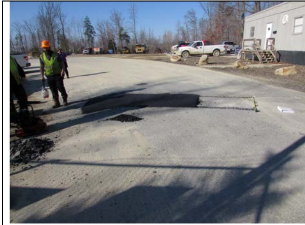
Figure 2. Hot Mix on left, chiseled area Cold patch evaluation
