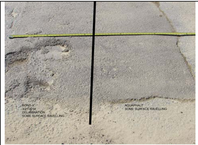
Figure 13. Bond-X delamination close up
