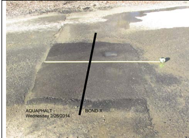
Figure 10. Patch loss of material
